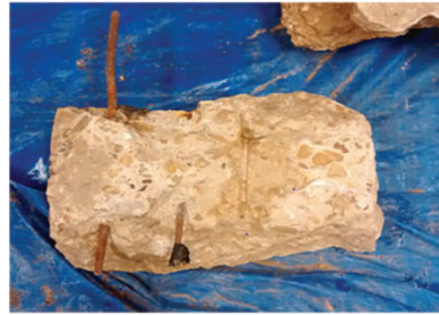
Figure 11. Specimen obtained from the IH-30 bridge deck
