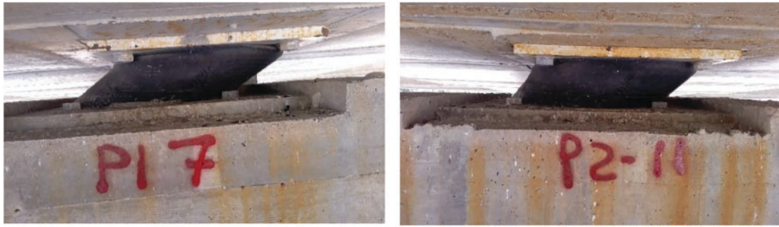
Figure 5. Permanent deformation observed on the HDRBs, after one year from the bridge construction
