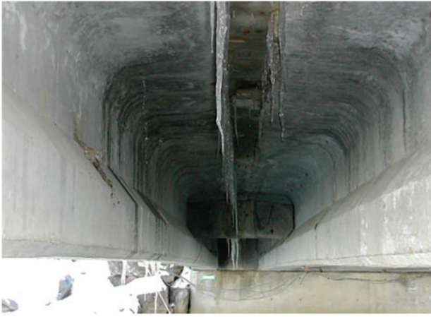
Figure 14. Icicles from water seeping between beams
