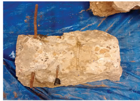
Figure 11. Specimen obtained from the IH-30 bridge deck
