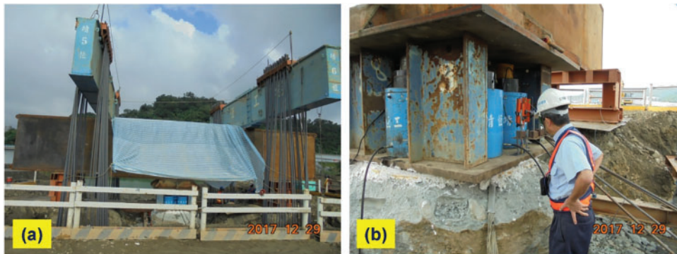
Figure 17. Testing equipment: (a) site test assembly and (b) monitoring instruments evaluated by the responsible engineer
