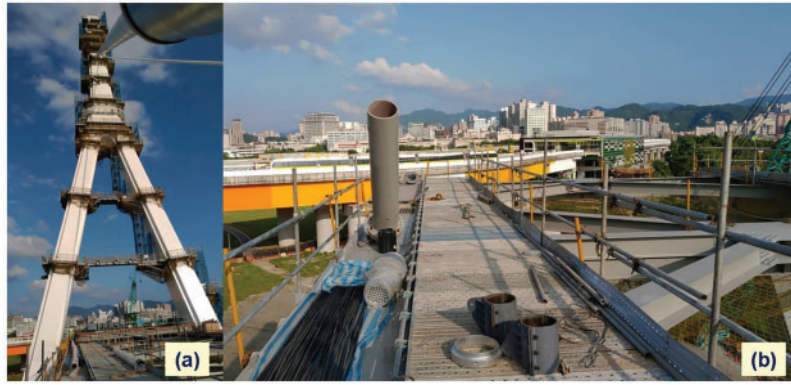
Figure 12. Site photographs of the safety facilities: (a) external stairs and temporary platform and (b) catwalk with the safety guard rails
