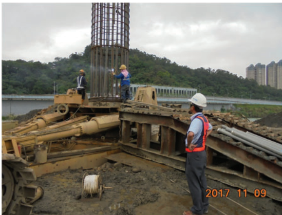
Figure 13. Rebar cage welding of the pile under the supervision of the responsible engineer
